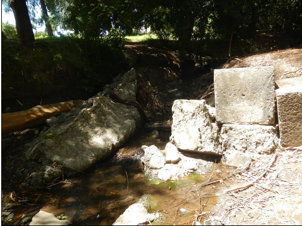
PHOTO 1. Failed Check Dam #1
