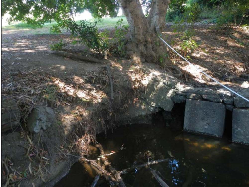
PHOTO 3. Erosion on Right Bank
