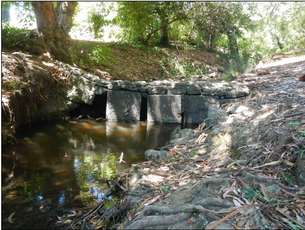
PHOTO 2. Failing Check Dam #2
