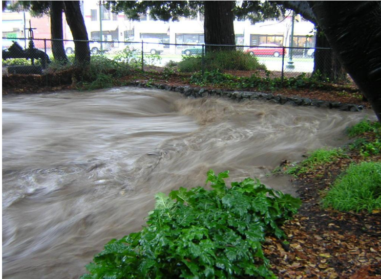
Backup at Oxford Street culvert during storm event February 25, 2004
